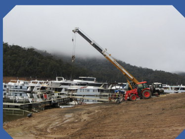
Fixing C Marina in July with a little help from a crane from Alexandra Cranes.
