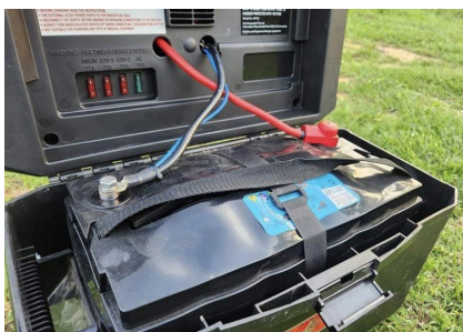
An AGM battery melt down. I am unaware of the cause but it's likely a charging issue. This just highlights that all batteries can fail when not adequately protected. A quality Lithium battery's BMS helps to protect itself from failure.
